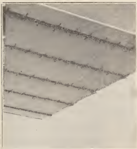
4. Soffit of corridor duct ready to plaster. Note spikes inserted thru holes in T-Irons at 6" centers. Soffit of duct only side built, ceiling and side walls of corridor acting as other 3 sides.
